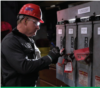
Operator Danny Roberts works on a temporary power supply panel during the Unit 4 outage.
